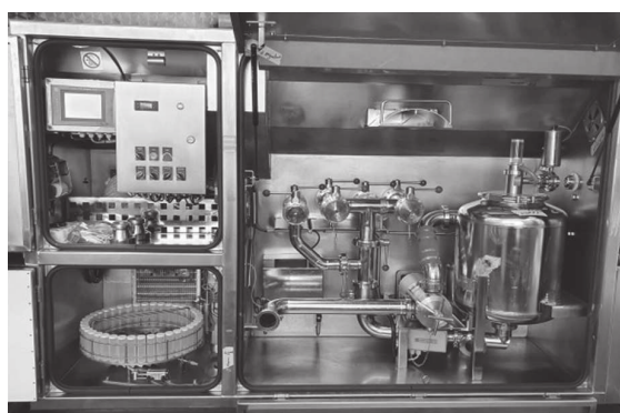
Figure 11. Cabinet interior with installation for milk collection and analysis at the tanker
